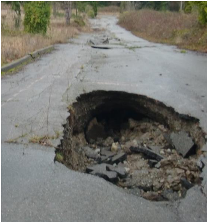
Sinkholes from failed CMP
