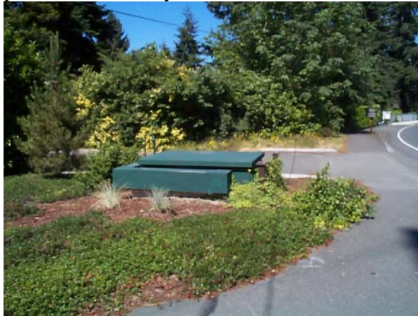
Underground Equipment Enclosure
