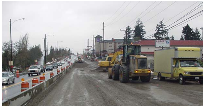
International Boulevard Phase IV work being done near S 208 th Street (funded by WSDOT). The profile of IB is being raised to avoid further disruption when the future SR509 crosses under International Boulevard.
