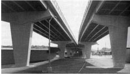
Figure 1: A Simple and Consistent Bracing Pattern with Uniform Girder Spacing Reduces Visual Clutter.
