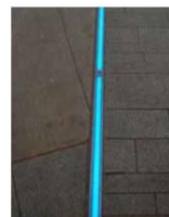
linear pavement lighting
