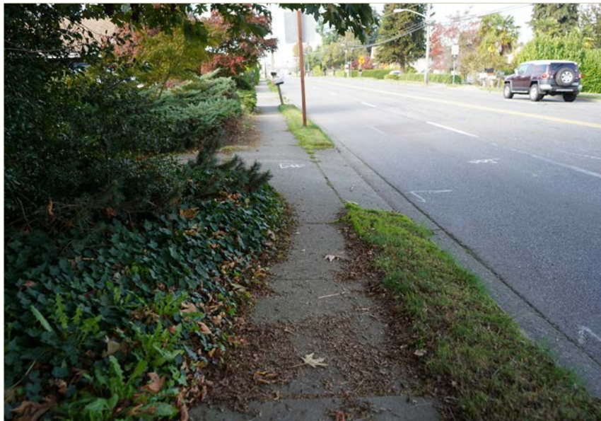
OVERGROWN VEGETATION NEAR MILITARY ROAD SOUTH/I-5/SOUTH 200 TH STREET
