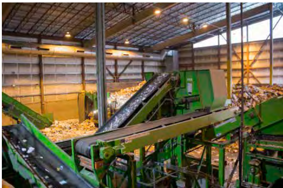
Recology CleanScapes materials recovery facility
