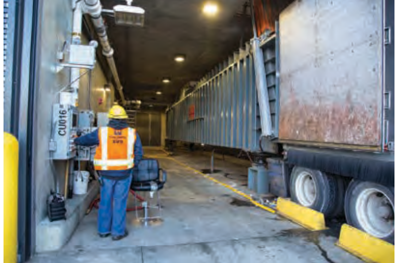
Compactors at the Factoria Recycling and Transfer Station compact trash, reducing the number of trips that county transfer trucks make to Cedar Hills
