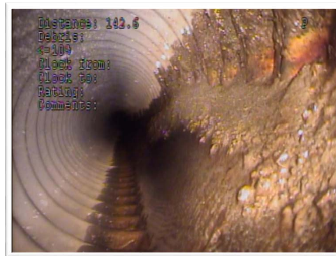
Erosion of Pipe
