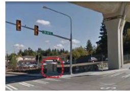
Traffic Signal Boxes - 192nd & IB
