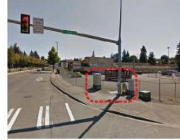
Traffic Signal Boxes - 28th & 192nd
