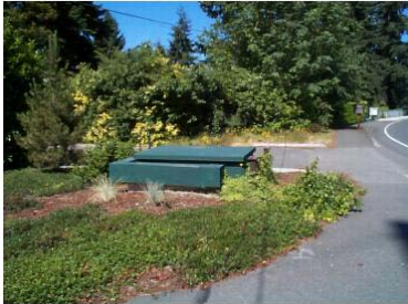
Underground Equipment Enclosure
