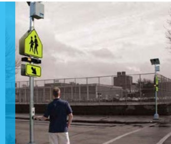
RECTANGULAR RAPID FLASHING BEACON (RRFB)
