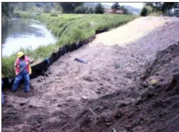
Silt fence being installed on a temporary access road; used as perimeter protection
