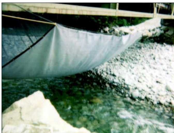
Diaper netting under bridge
