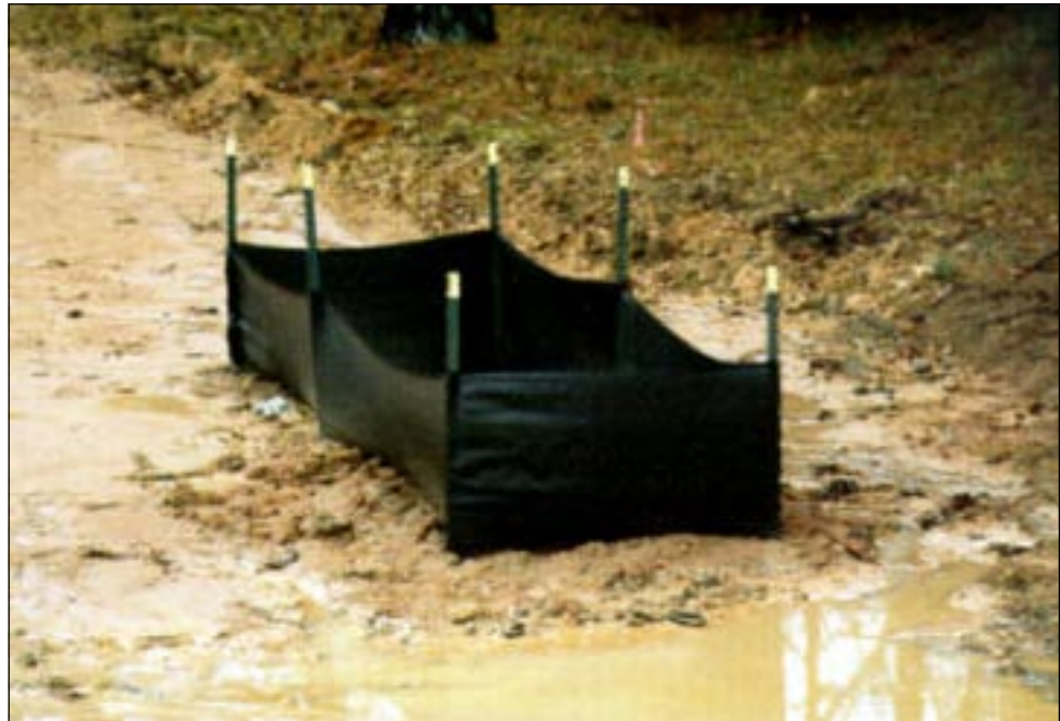
Inlet protection: filter fence surrounding catch basin to reduce soil particles from entering drainage system
