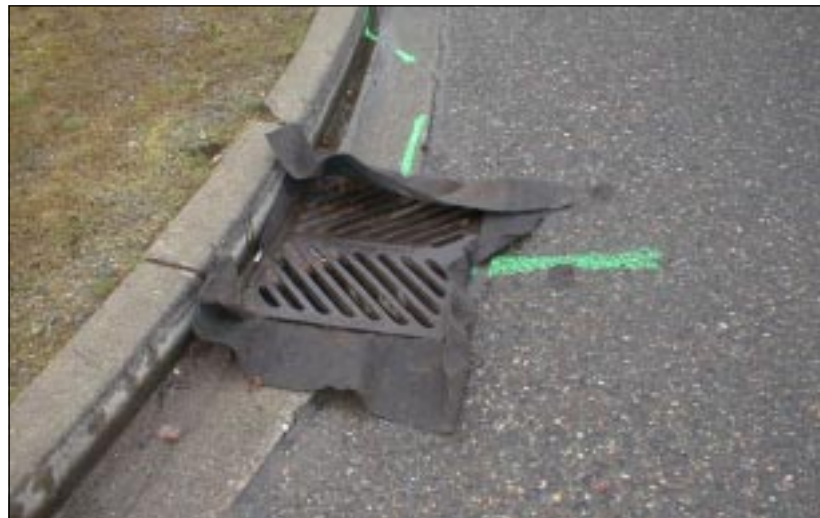
A silt sock installed in a catch basin to trap/filter waterborne soil particles
