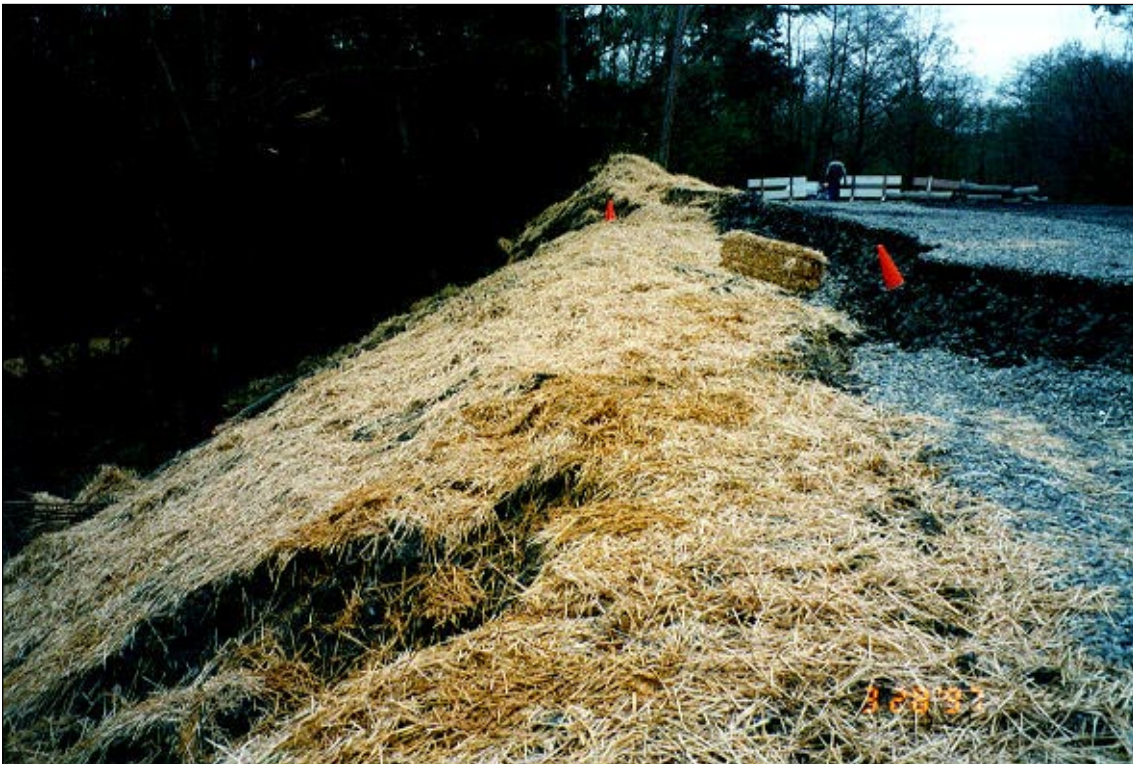
Using straw to reduce erosion in a slide area prior to a major stabilizing project
