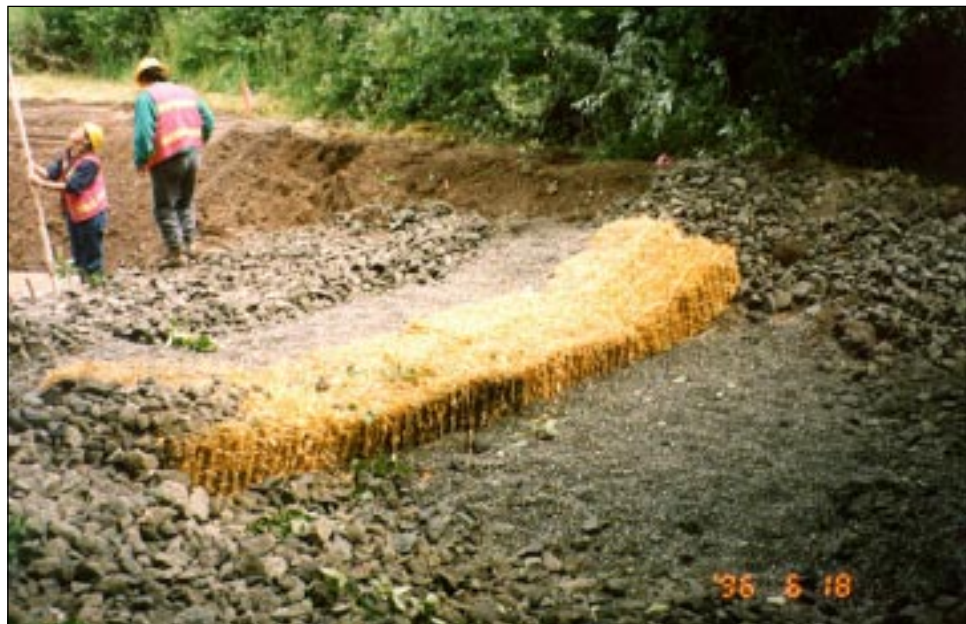
Straw Bale Barrier (3) being used with a rock spillway decreasing runoff velocity and retaining sediment onsite
