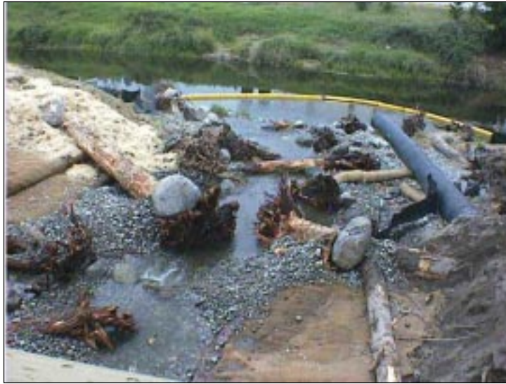
Large woody material placed in a streambed to provide salmonid refuge. Note use of turbidity curtain, streambed gravel, silt fence, coir fabric, mulching, and stream bypass
