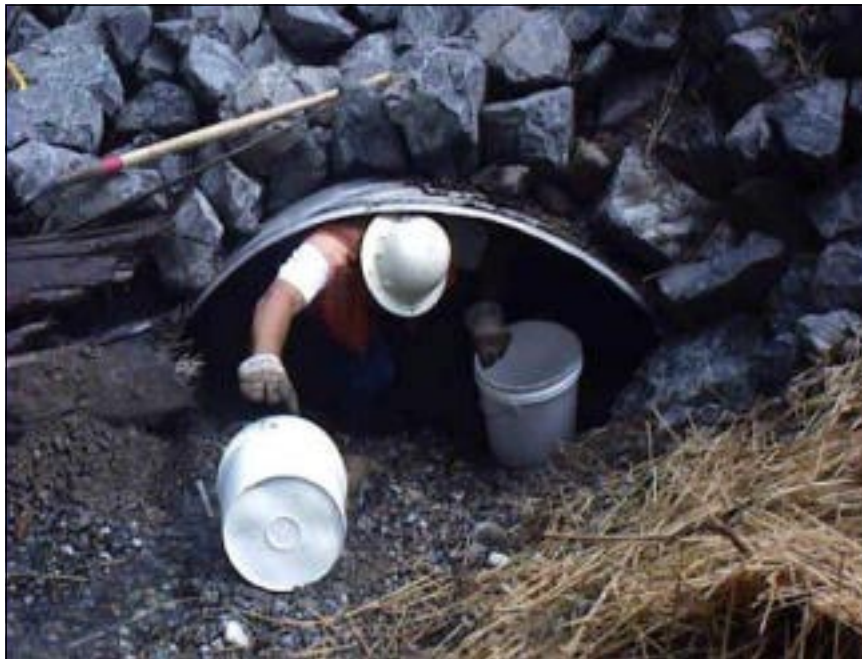
Placing streambed gravel inside a newly installed cross culvert to provide a natural substrate for fish
