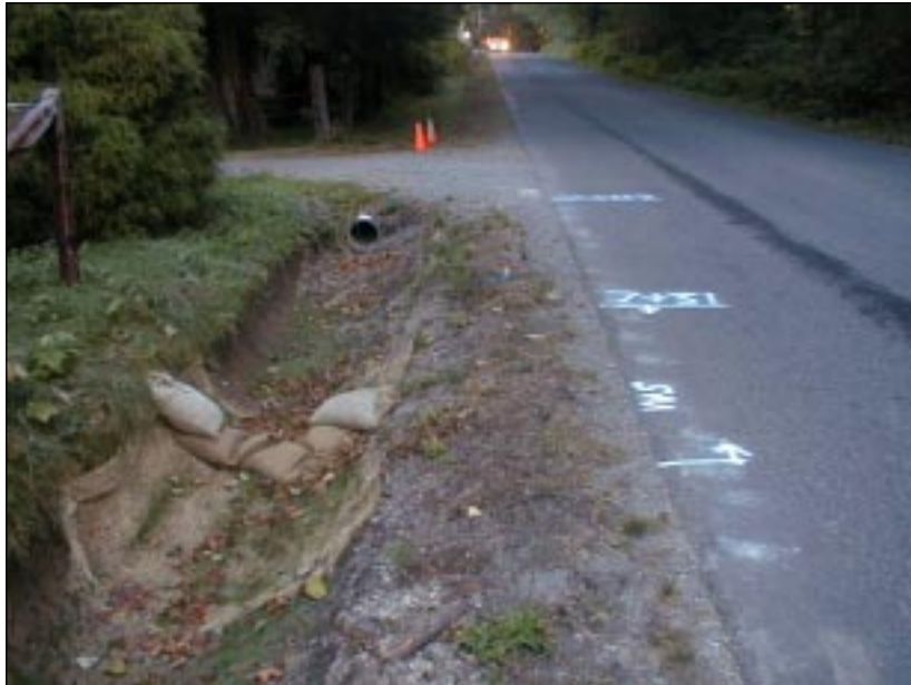
A sandbag barrier used to decrease water velocity. Note use of silt mat and hydroseeding to decrease erosion and to increase vegetation in channel
