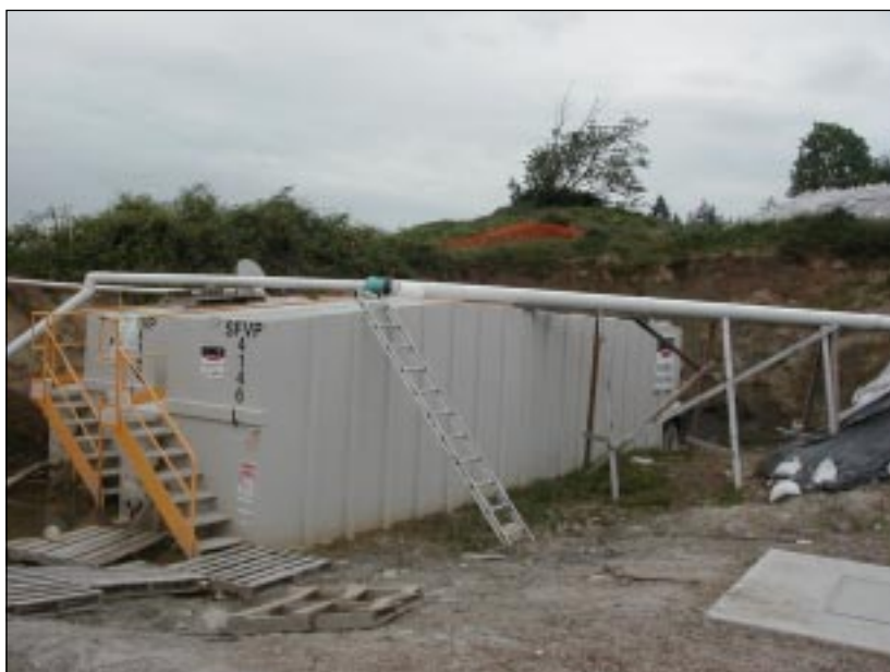
A settling tank in use to allow onsite containment of water borne soil particles
